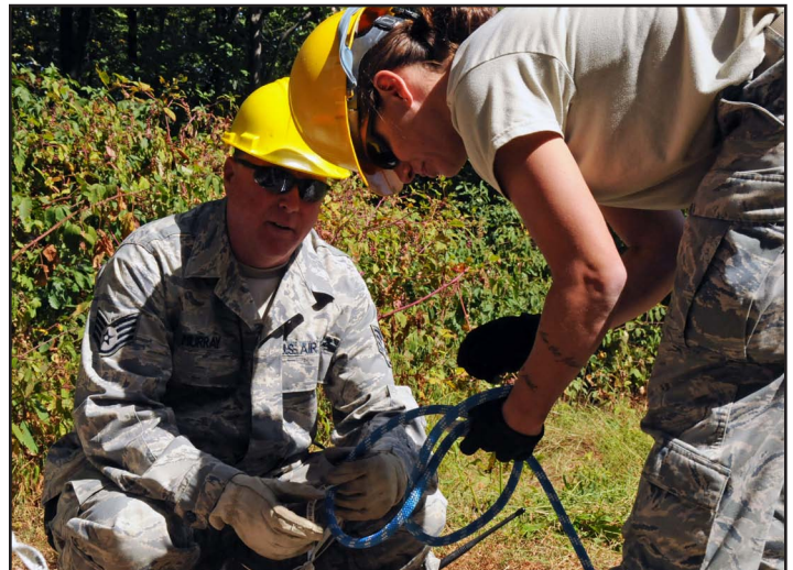
Staff Sgt. Charles Murray and Airman 1st Class Christian Dolbin, both 211th Engineering Installation Squadron, cable and antenna installers, work to secure a line to the VHF antenna so that it can be transported up the tower where four Airmen wait to attached it to the mast they installed. (Photo by Senior Airman Claire Behney)
